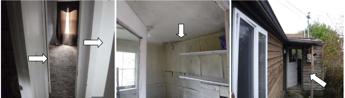
Photos 4-6: Representative Photos of Lead-Containing Paint on Wood Trim and Plaster Walls at Southwest Bedroom and Hall (L), and Cream Paint on GWB Walls (C), and on Wood Door and Trim Components at North Exterior Utility Room (R):
