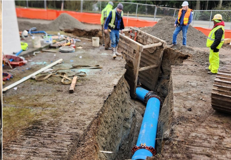
New forcemain at Pump Station 4
