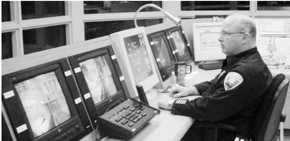
Corrections Officer Dave Rash controls prisoner movement and monitors housing unit activity from the jail's new computerized Central Control station.
