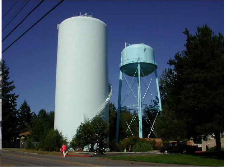
1721414 – Elevated Steel Tank and Welded Steel
