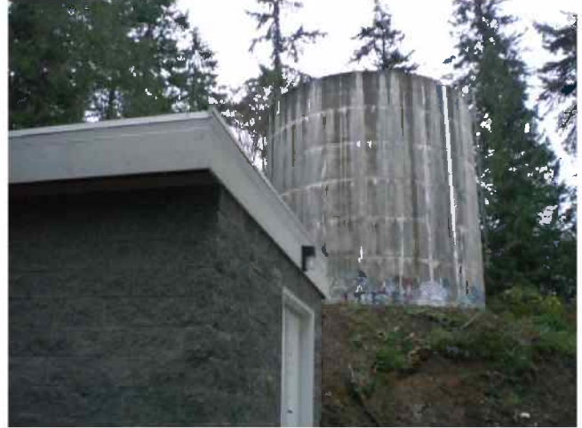
2175727 – Concrete tank with Shed-GP
