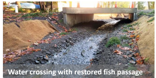
Fish passage barrier due to low water depth
