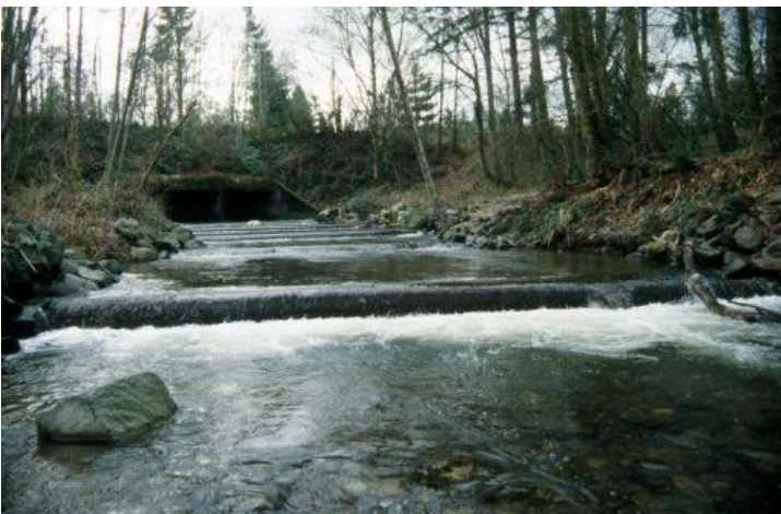
The log weir fishway at the outlet of the Golf Club Hill Road culvert caused additional impacts.
